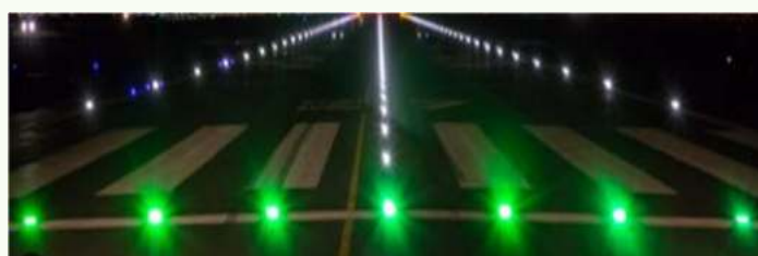
Threshold Lights (green)
